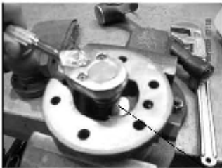
Remove and inspect pilot seal & pilot strainer.
